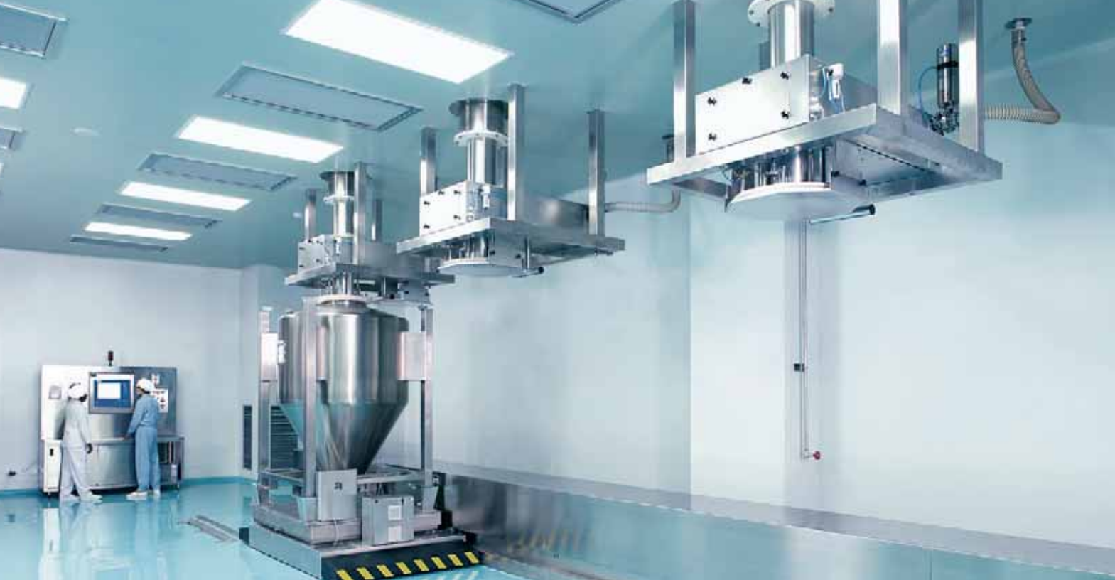
Automated collection and weighing of the components by an AZO COMPONENTER®
