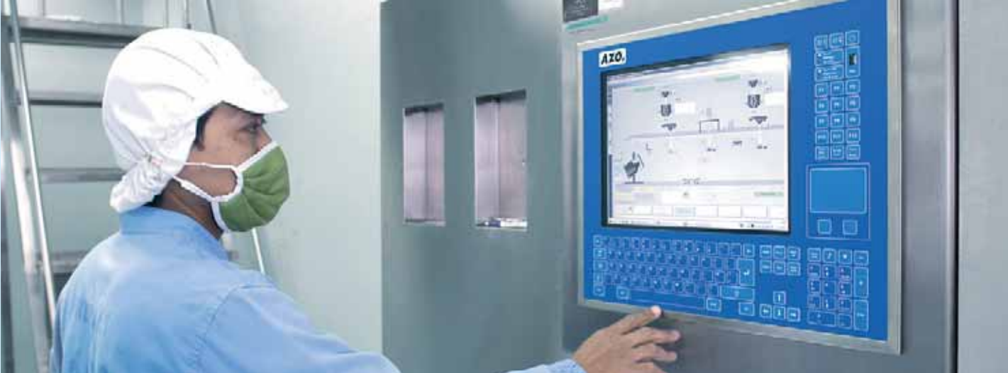
Operator control terminal on-site
