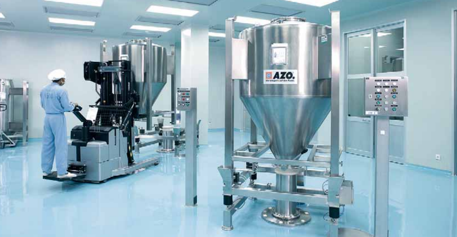
BATCHTAINER® with finished mixed product for feeding the tablet presses on the below level
